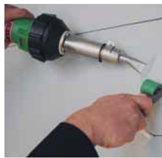
Using the TRIAC PID to weld a patch on a building site.
