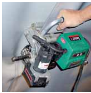
TWINNY T with convenient cross-handle at work: overhead welding in a tunnel.
