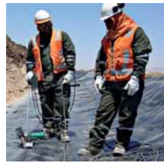
TWINNY S with combi-wedge at work at a mining site in South America.
