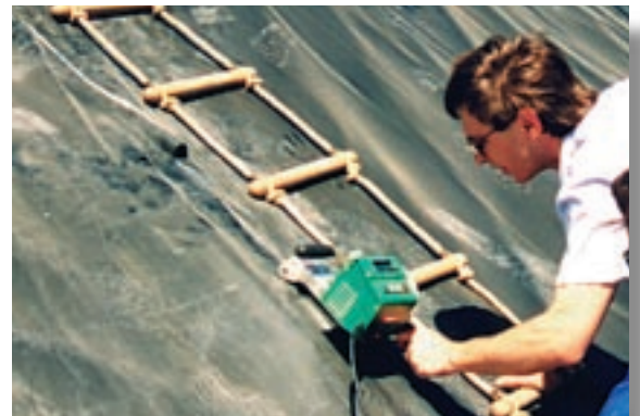
COMET wedge welding machine used for welding geomembrane liners in a landfill.
