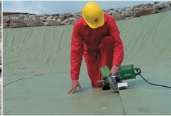
TWINNY T used in a water storage basin.
