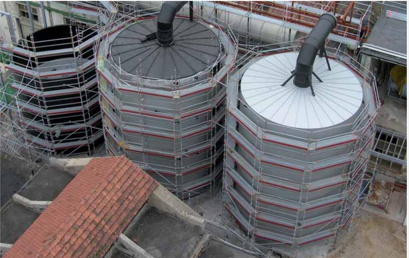
40 feet high silos was made of HDPE, Spain. (Photo: Colasit)
