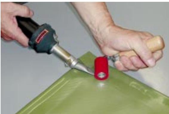
HOT-JET S with wide slot nozzle and pressure roller used for welding a billboard.
