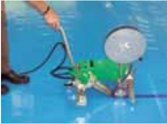
A 40 mm reinforcement tape is welded with UNIMAT TAPE onto a PVC sheet.
